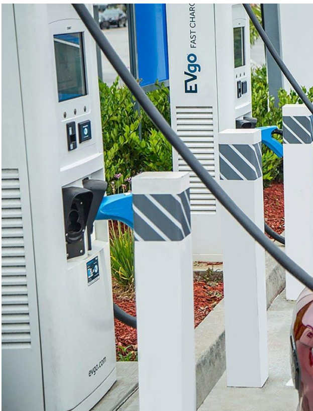
Photo: Oklahoma Commercial EV Charging Stations
